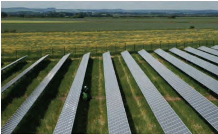
Figure 6 Adequate spacing between rows of panels is necessary to avoid overshadowing. Vegetation will grow between these rows and this vegetation will require management.
