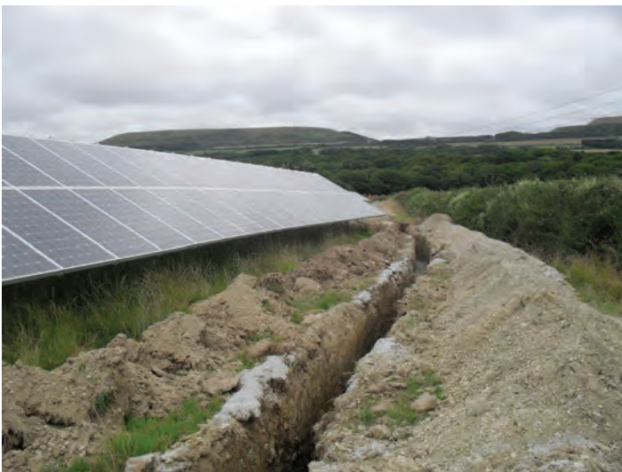
Figure 9 Soil excavation during cable trenching at the 5MW Trefullock solar farm in Cornwall. Note how topsoil and subsoil are stored on opposite sides of the cable trench in order to avoid the mixing of soil types and facilitate subsequent soil replacement and site restoration.
