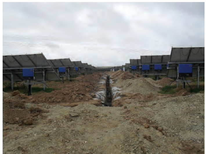
Figure 10 The construction compound associated with the development of the 5MW Trefullock solar farm in Cornwall.
