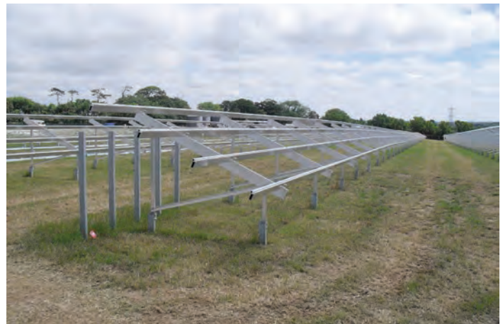
Figure 14 The ground anchors and framework associated with the development of the 1.4MW Benbole solar farm in Cornwall.
