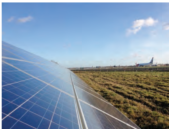
Figure 23 Solar panel array at Gatwick airport. Image courtesy of Orta Solar.
